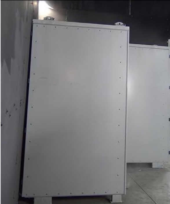
(e) Cell 21 thermal runaway [00:44:19]
